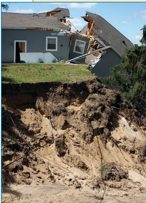
The soil under this house has been eroded away.
